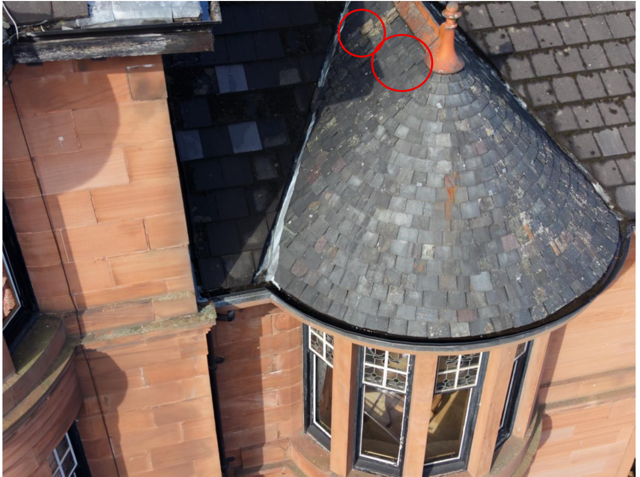
Image 4 (Left bay window, left side) Image shows at least 2 missing slates
